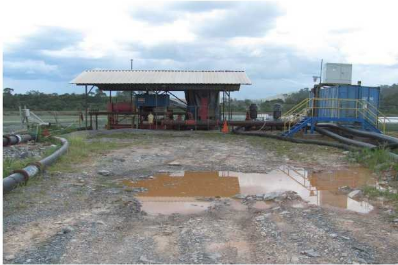
FIGURE 18-3 FIRE PROTECTION PUMP FACILITY
