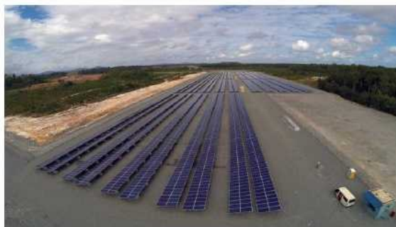
FIGURE 18-4 ROSEBEL 5 MW SOLAR POWER PLANT
